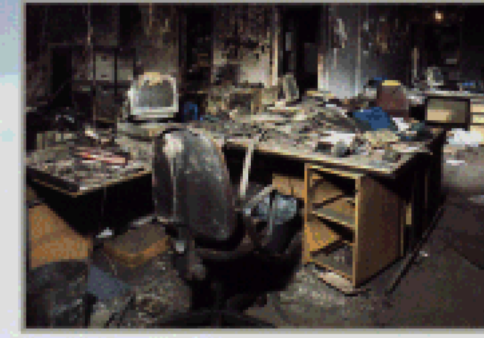
A damaged office by fire A damaged computer can be replaceable but damaged data can't be recovered.
